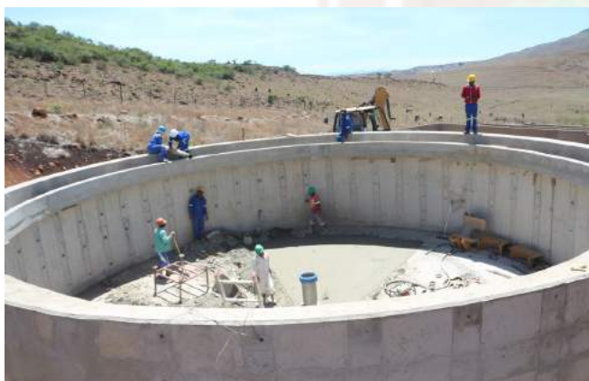
Above: Construction of waste water treatment works in progress in Ntabankulu Local Municipality
