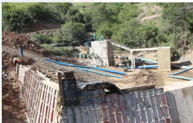
Above: Bomvini / Nyokweni water scheme which expected to bring credible water to Ntabankulu communities
